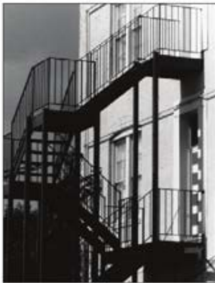
Above: The placement of fire escapes at the rear of buildings usually is appropriate.
