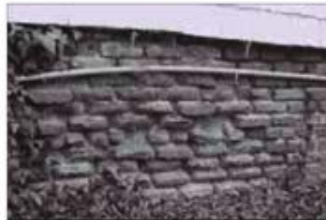
Mortar joints should be kept in good repair. Significant moisture damage is evident in this photograph.
