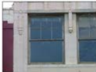
Historically, windows were true divided lights in nature. Traditionally, most windows installed during the period of Aiken's primary downtown commercial development were 1-over-1, or 2-over-2 in pattern. However, installations such as the 6-over-1 pattern shown above were used successfully to introduce character and variety.
