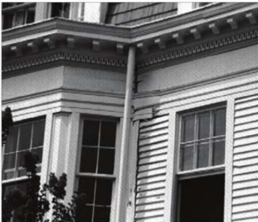
Damage to exterior wood was probably caused by gutters and downspouts that were leaking or that were not cleaned frequently.
