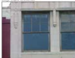
Historically, windows were true divided lights in nature. Traditionally, most windows installed during the period of Aiken's primary downtown commercial development were 1-over-1, or 2-over-2 in pattern. However, installations such as the 6-over-1 pattern shown above were used successfully to introduce character and variety.
