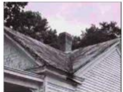
This chimney (above) probably is brick with a corbeled cap. The stucco was probably applied in lieu of repointing and detracts from the original character of the building.
