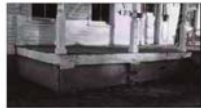
The acceptable brick enclosure (top photo) was "pierced" to allow for air flow under the building. While the infill (bottom photo) was recessed to emphasize the original brick piers, the lack of ventilation is inappropriate.
