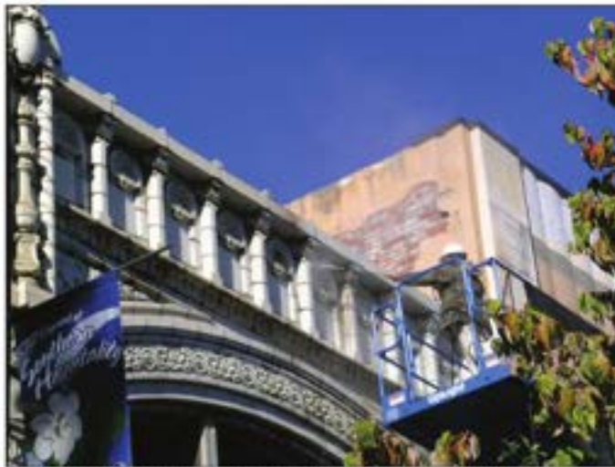
terse colts cornice cleaning via a low-pressure water wash and mild detergent.
