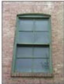
True divided light wood windows were the norm in traditional construction. 4-over-4 pattern.
