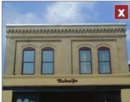
In this example, the original arched-top windows were removed and rectangular units were installed in their place with a wooden "filler" inserted in the arched area. This gives the appearance of an "eye lid" closing above the windows. Always fill the opening with an appropriately sized window.
