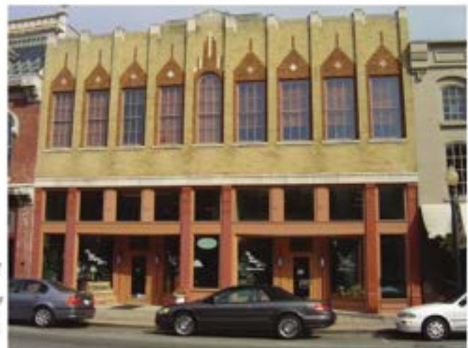
Examples of traditional storefronts show the various parts of an entry way including transom windows, recessed doors, and display windows.
