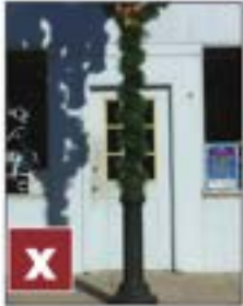
The style and detailing of this door is inappropriate to the building itself and the overall character of the district. The door utilizes a window and panel system that would have been associated with a "colonial" style building, not the Victorian/Commercial style of downtown Aiken.
