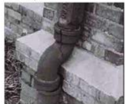
Below: The missing and damaged portions of downspouts should be replaced.
