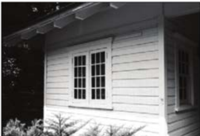
Each board of drop siding (German, shiplap, or novelty siding) has a rounded channel above a flat surface.
