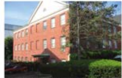
This side facade shows blanks used in place of actual window openings to continue the established window pattern in locations where windows were not feasible.
