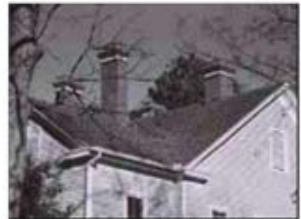
The number and style of chimneys are important indicators of the age of a building.
