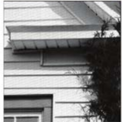
Installation of substitute siding changed the appearance of the building shown above. Because of the vinyl siding and probably a thin layer of insulation beneath it, the window frame and cornices are recessed instead of slightly projecting. Soffits are no longer smooth wood. If peeling and blistering paint led to the siding installation, the siding may be trapping the moisture that caused the paint problems and creating an ideal environment for decay and wood-loving insects.
