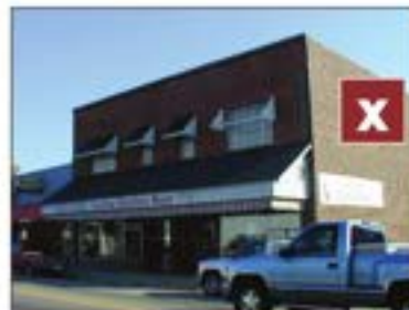
The shingled "roof" awning/canopy is inappropriate to the scale of the building & conceals the upper facade.
