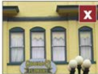
The windows installed in this existing building are inappropriate. They should relate to, and fill, the entire arched opening in the masonry above.
