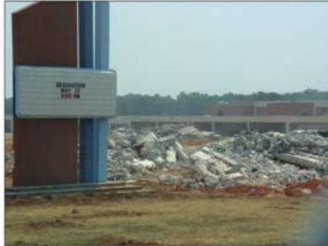
Occasionally, demolition is the only course of action that remains for a property. A plan for the site's reuse is a critical component in the evaluation of a request for demolition.
